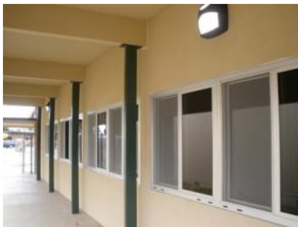
Bayside Elementary – Newly installed windows at Bayside Elementary will allow for more daylight in the classroom, significantly enhancing the learning environment for students
